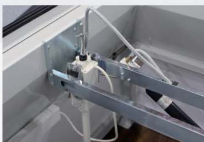
Separate motor for ventilation purposes
